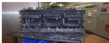
Fig2 .Damaged due to overheating cluster
